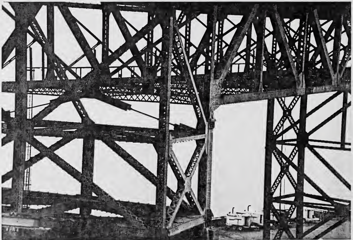
and it is a group of us climbing the steel truss (lower part of bridge) to the catwalk . . .
